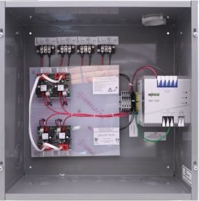
AFI RQ Control Panel Integrated to BAS via BACnet/MSTP. Custom configured multi-channel units Up to 12 actuators per Panel
