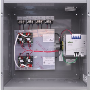
AFI RQ Control Panel Integrated to BAS via BACnet/MSTP. 4 Channel 12 Actuators per Panel
